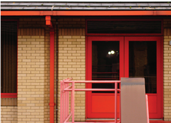
Figure 54. Example of poorly located a down-conductor.
