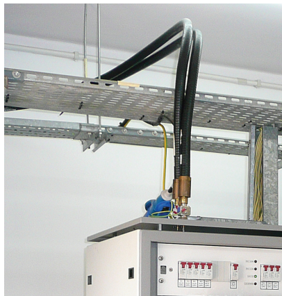
Figure 113. Incoming antenna circuits require protection.
